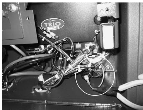
Figure 1 Jumper wire disconnected
