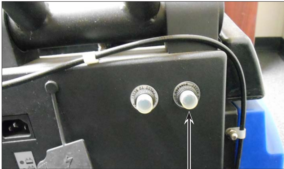
Brush Circuit Breaker
