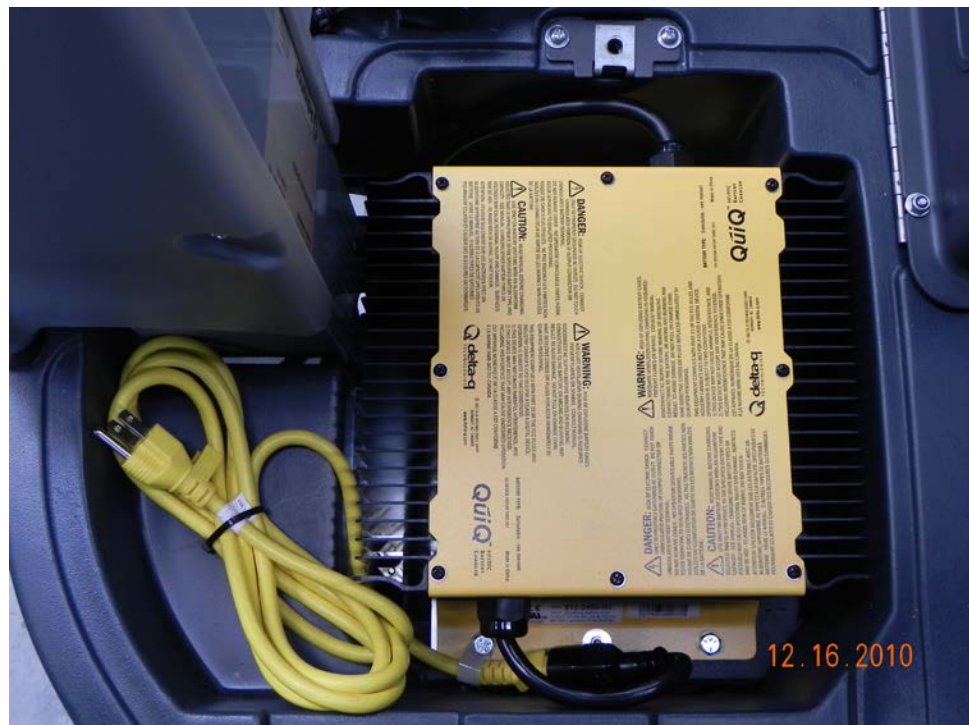
Battery Charger with AC power charging cord
