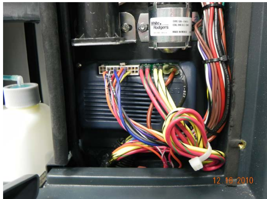
Speed Controller - Located under Electrical compartment
