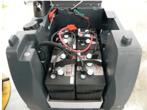
Batteries in battery tray with Recovery Tank removed and Operator's Seat up.
