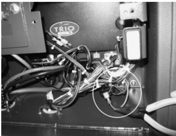
Figure 1 Jumper wire disconnected
