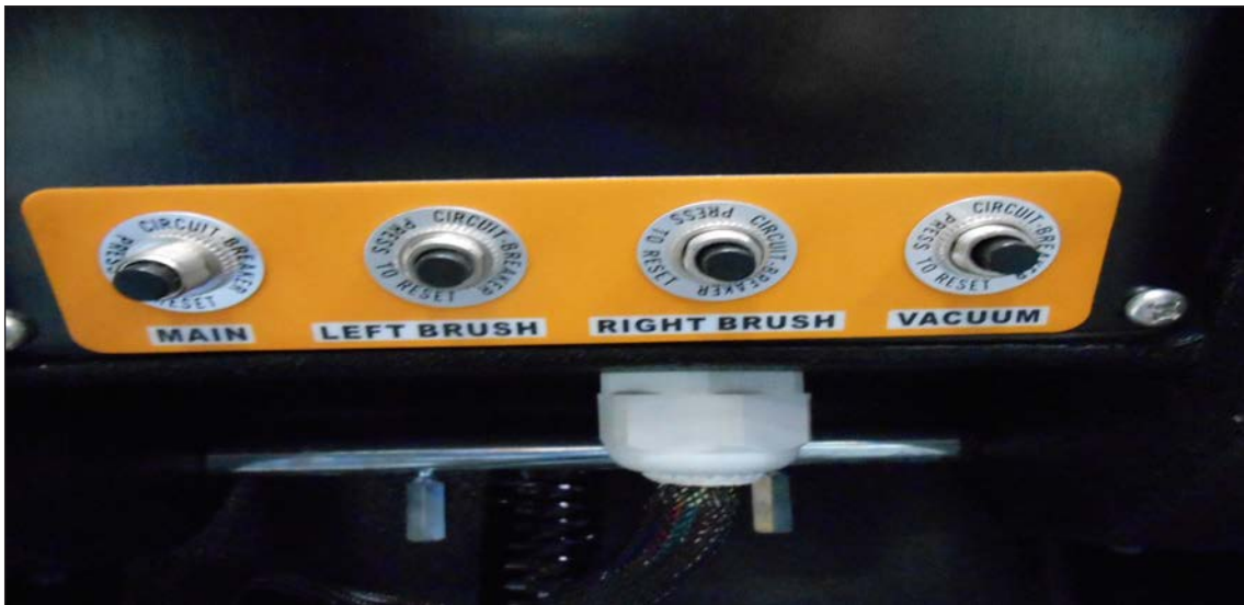
Circuit Breakers (Located on lower control housing panel)
